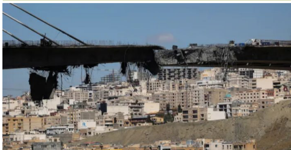
The B1 bridge was damaged in U.S.-Israeli strikes in Karaj on April 3, 2026
